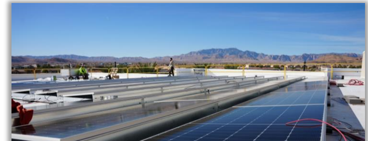
Southern Nevada Solar Projects at our Corporate, North & South Facilities
